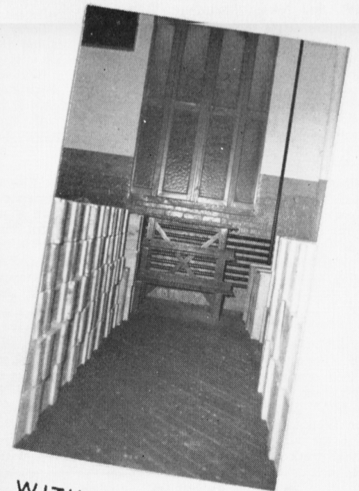
WITH FIRE ESCAPES CLEAR, NO DANGER
